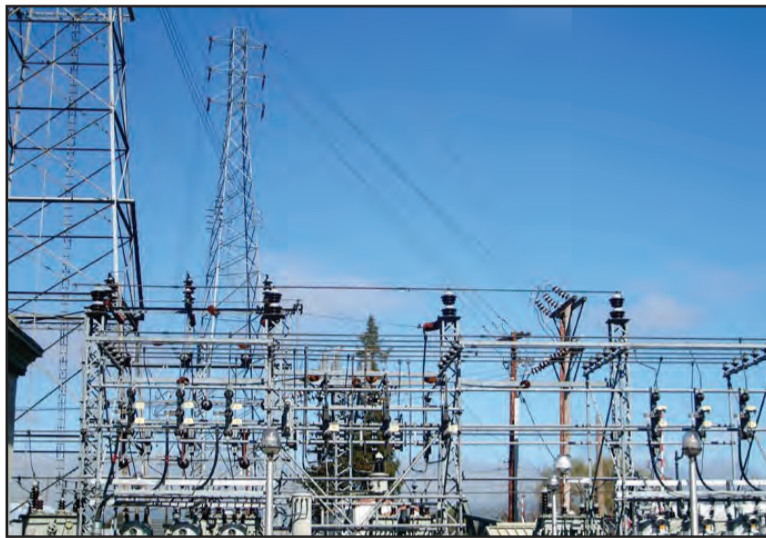
One of the power stations that ensures the stable supply of electricity to households and industries in the city.
