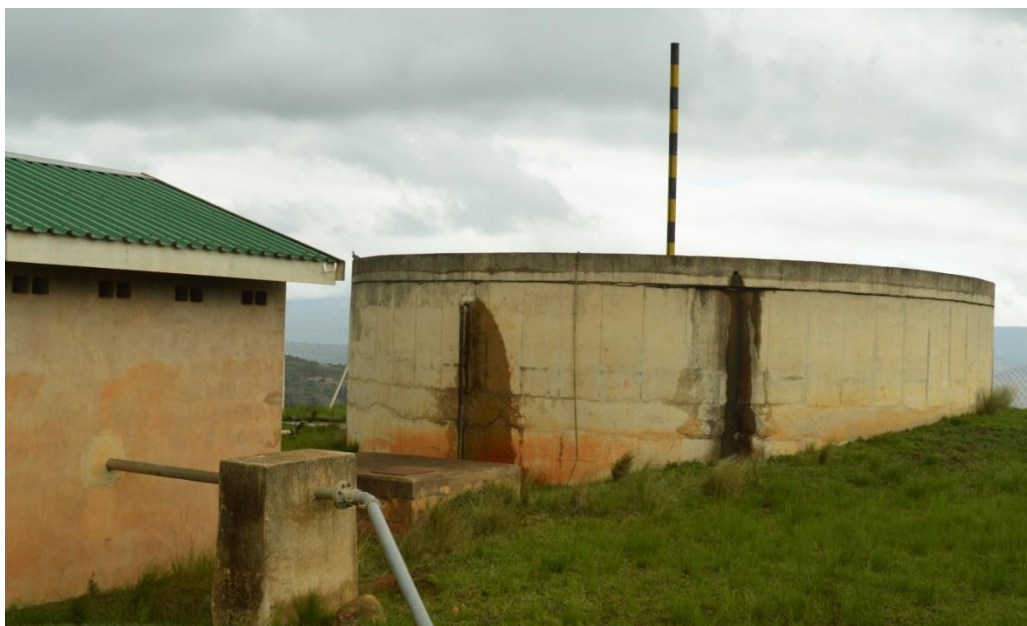
Figure 82: Reservoir above the Ncwadi clinic
